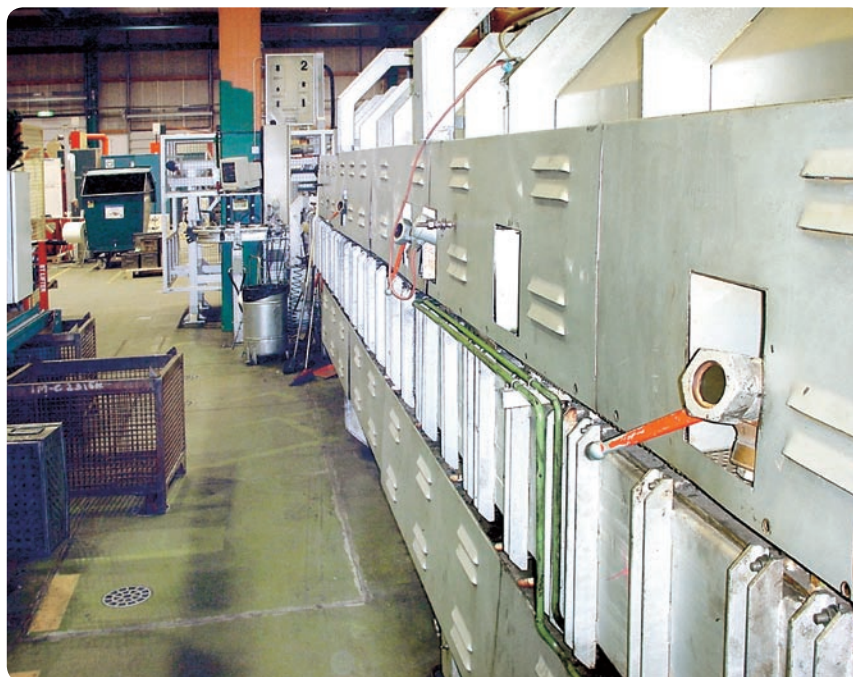
Heat treatment oven at SKF equipped with high-temperature bearings
